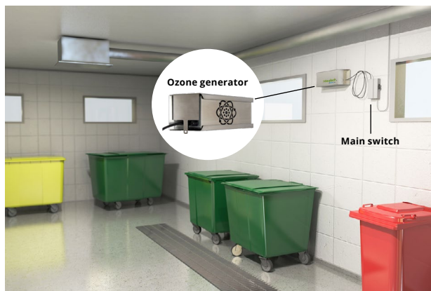
The ACT 3000 ozone generator is mounted on a sturdy wall bracket and the ozone production control is easily accessible.
