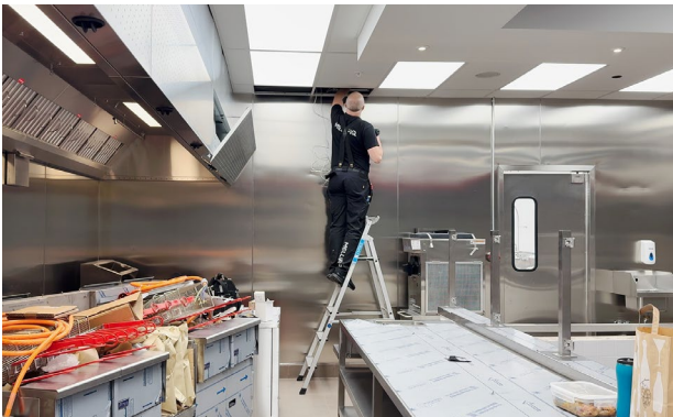
Setting up the RENA system, with integrated ozone injection in the ventilation.
