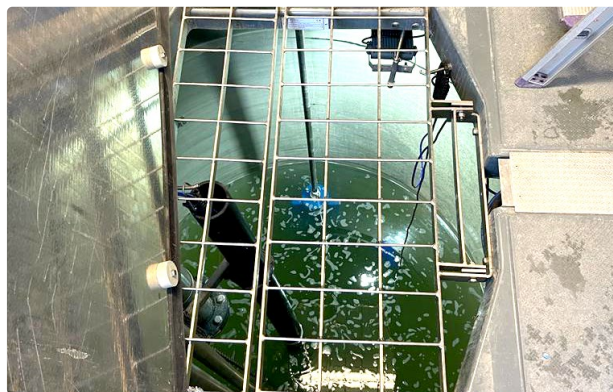
API removal plant pump station, designed and installed by Mellifiq.
