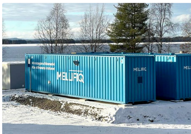
Advanced quaternary treatment stage for pharmaceutical residues installed in two 40' containers, specifically engineered to operate year-round
