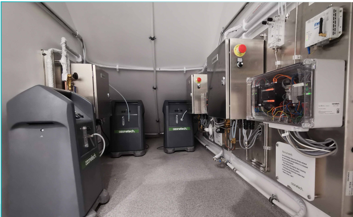
View of the installed Ozonetech RENA Commercial Kitchen Solutions.
