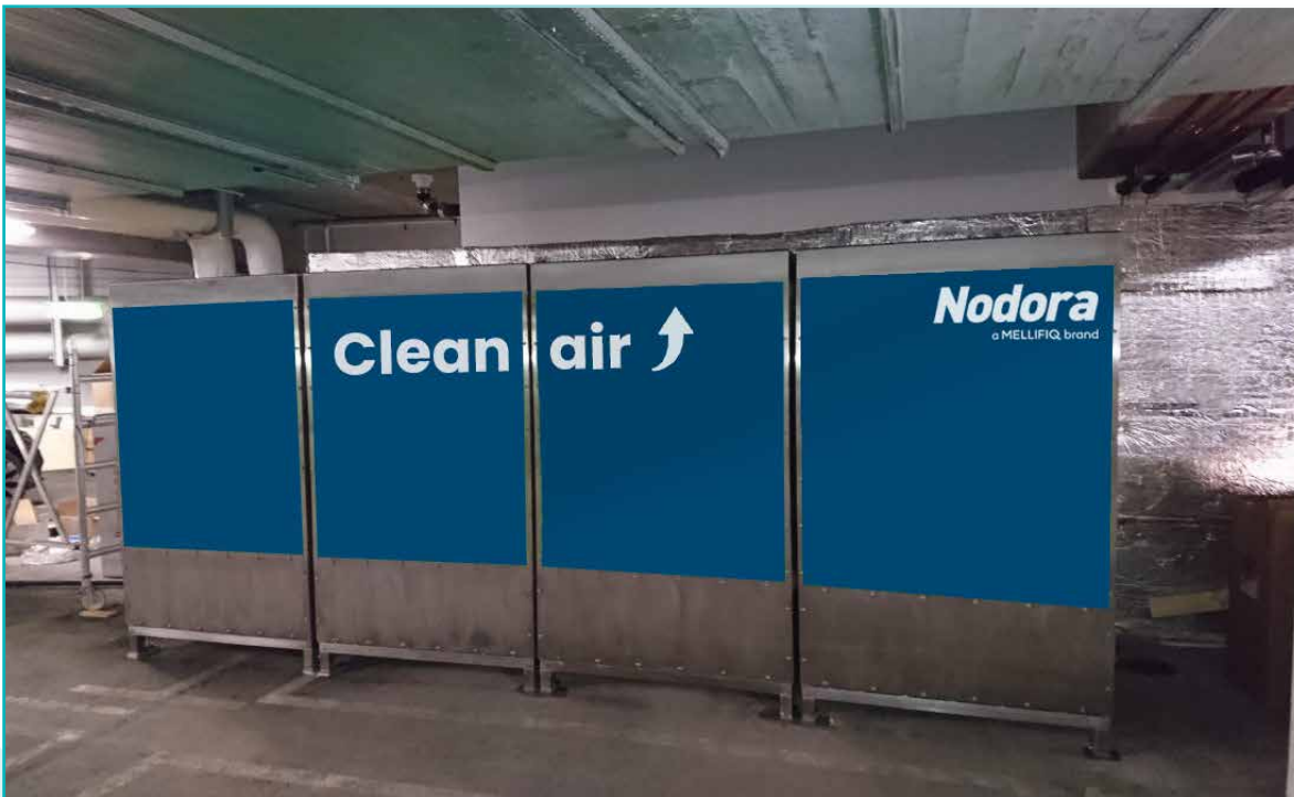
View of the installed Nodora ADS.
