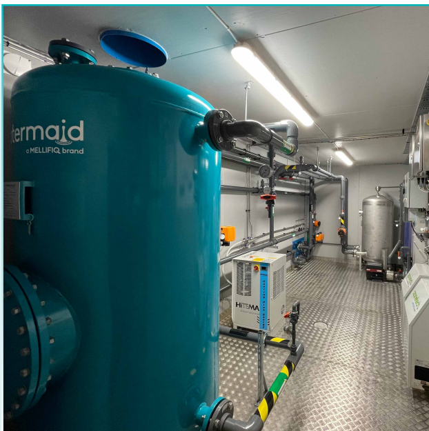
Image from the inside of the 20 ft container.
