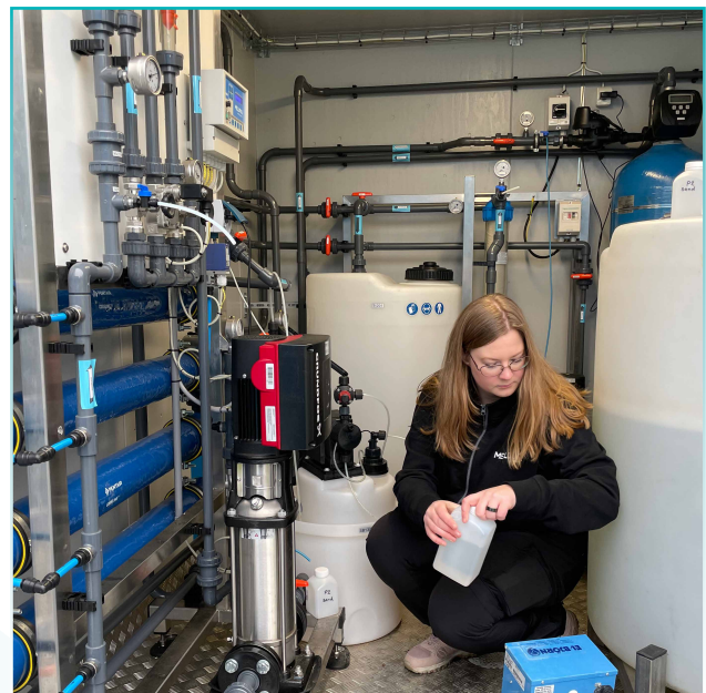
Image from the inside of the 10 ft container.
