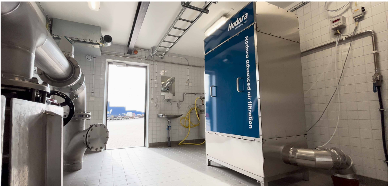
The installed Nodora CAT located in the pumping station.
