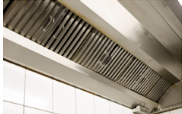
The air treatment takes place in the kitchen ducts above the frying surfaces. The fat particles are broken down in 3-5 seconds.
