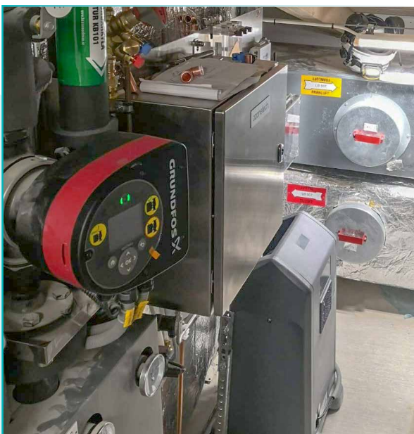
View of the installed Ozonotech RENA Commercial Kitchen Solutions.
