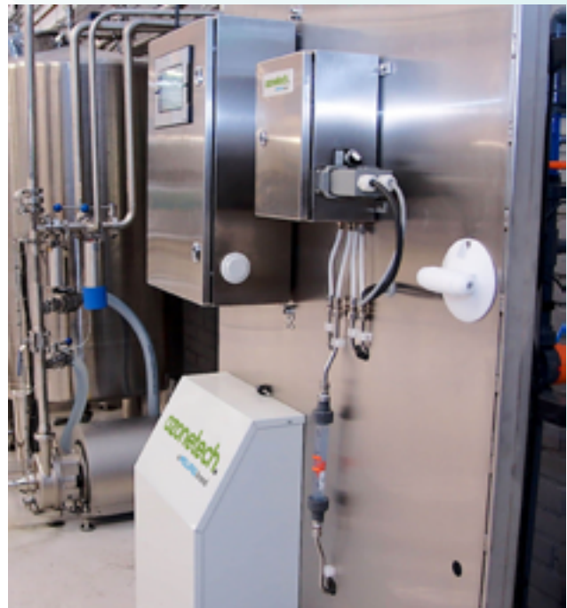
The RENA Vivo A-series is integrated into the existing CIP system.
