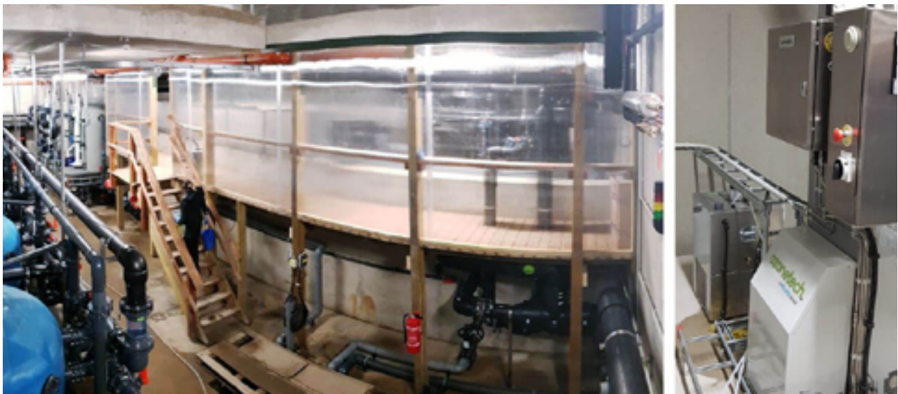
The ozone system was integrated into the new facilities from the start (to the left). The RENA Pro C6 system with integrated cooling system installed at Tallinn Zoo (to the right).
