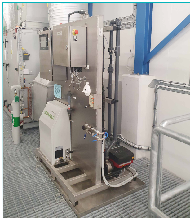
The Ozonotech RENA Vivo system installed on site.
